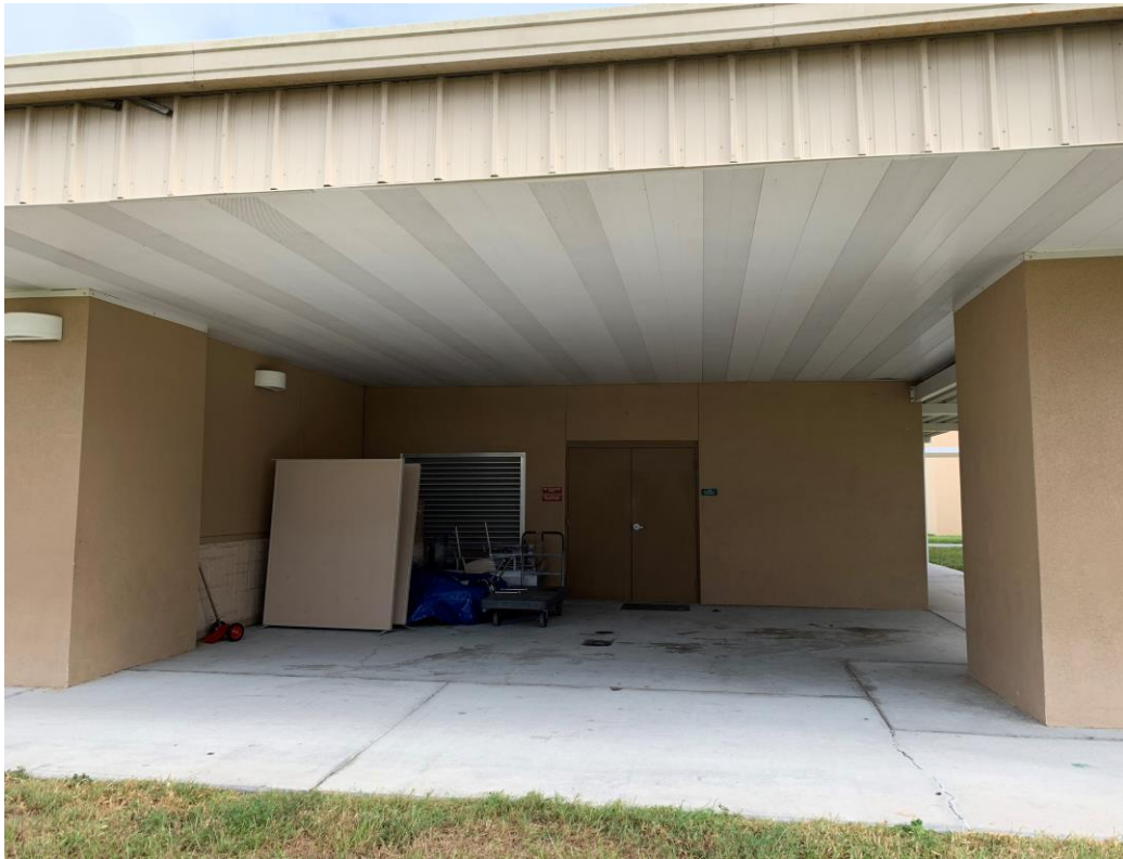
BELA- Enclose End of Building for Storage Project Pictures of the end of the 200 and 300 building.
